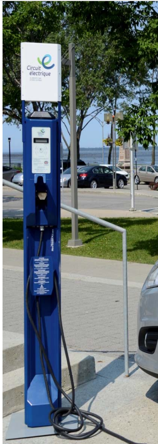
240V charging stations (600+ in service)
