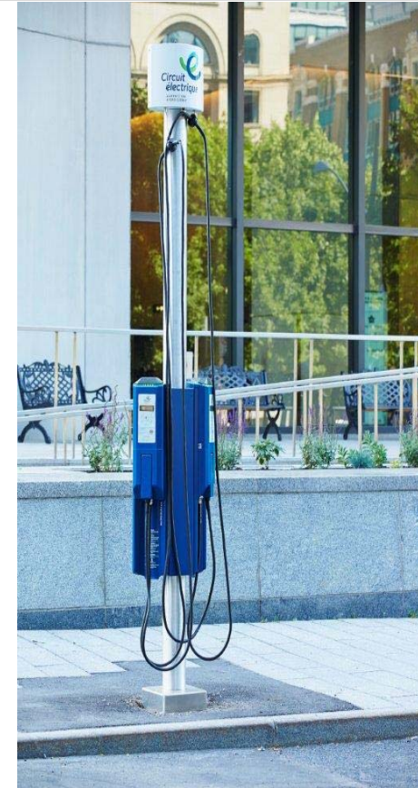
Curbside charging stations (20+ in service)
